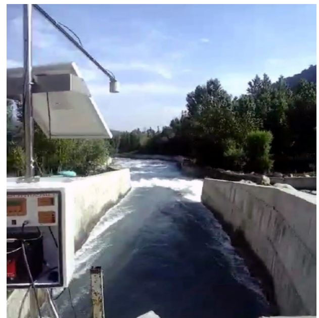
Installation at NHPC Jammu and Kashmir
